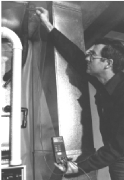
FIGURE 47 TEMPERATURE RISE MEASUREMENT
