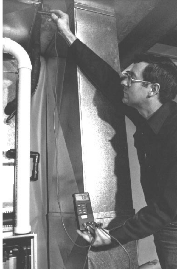
FIGURE 20 TEMPERATURE RISE MEASUREMENT
