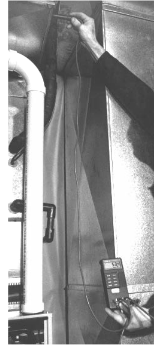
FIGURE 47 TEMPERATURE RISE MEASUREMENT
