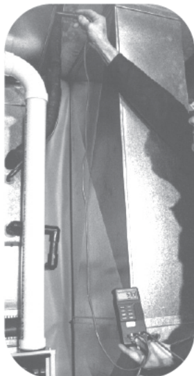
FIGURE 57 TEMPERATURE RISE MEASUREMENT
