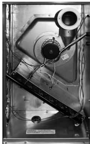
Heating Compartment Access
